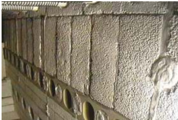
Fig.7: Wall area of a roller kiln with special pre-cast insulating bricks.
