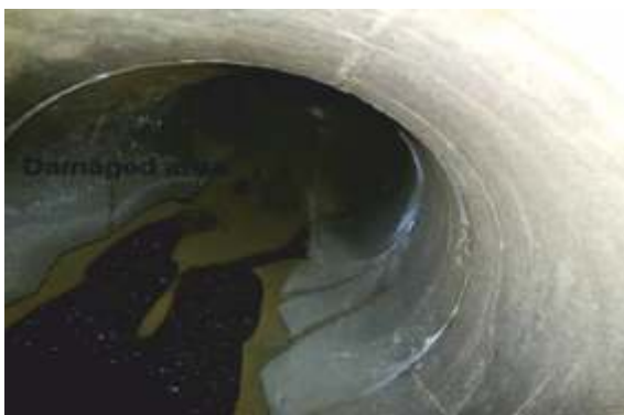
Fig.4 Ejector damaged after 15000 Tons production
