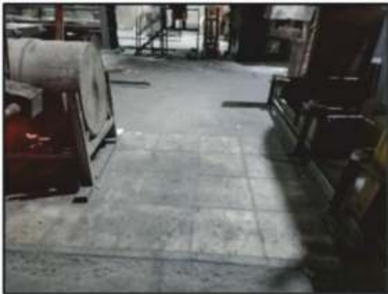
Figure 5: Image of a pre-casted area in the foundry facility in Nagpur prior to installing new flooring
